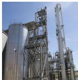
Ethanol production plant
