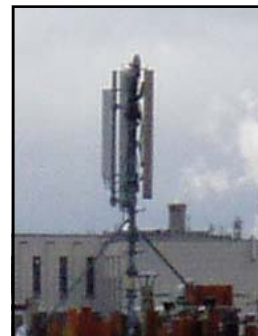
View of a mobile phone mast
